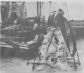
This is the Pump Body which actually does the dredging.
